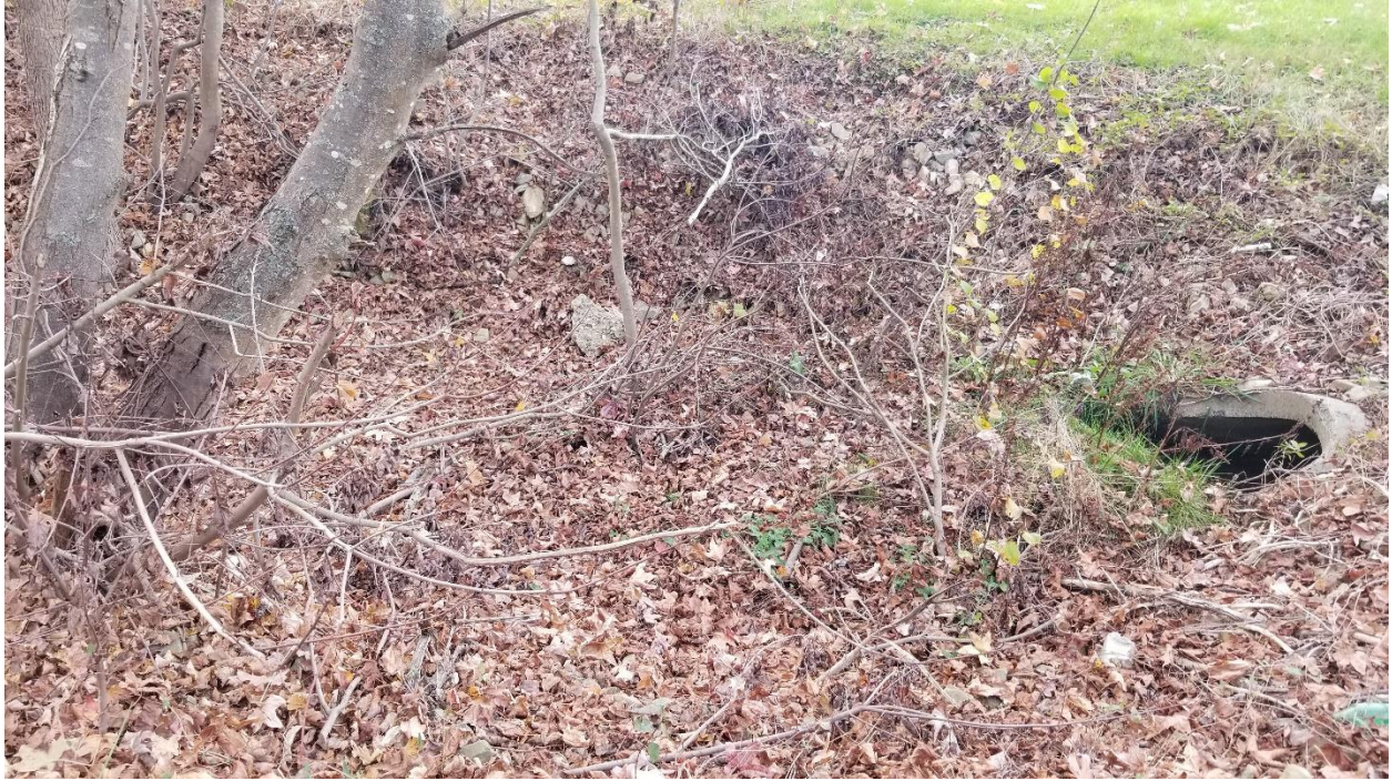
Photo 15 – Standing along Buck Road, across the street from the site, looking west at an existing pipe outfall.
